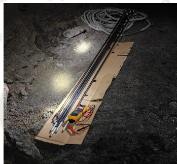
Fig. 4: Rock bolts with printed sensors in a mine
